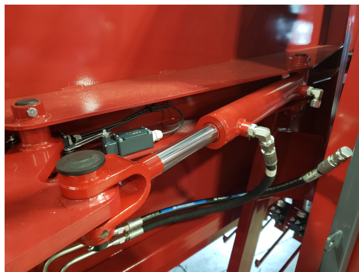
Example of a cylinder that has extended indicating a faulty seal on the piston
